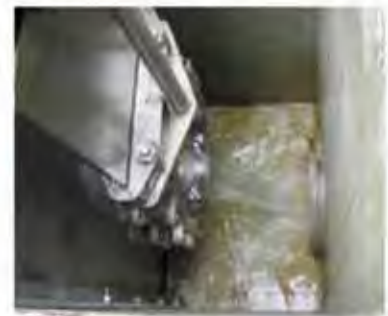
Emergency cutoff valve at the final discharge outlet
