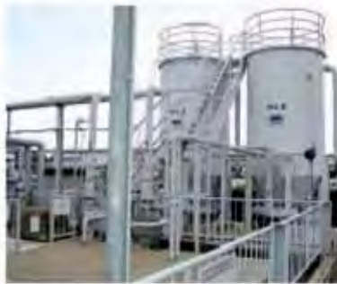
Waste water treatment plant sand filtration system
