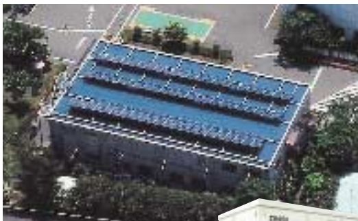
20kW solar power generation system at Term Corp.
