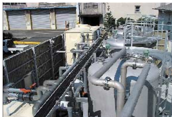
Pumped-water purification system
